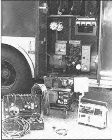
On-board and portable generators and lighting equipment.
