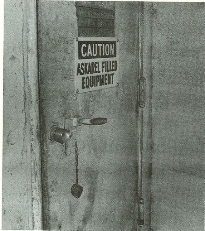
Warning sign on door leading to transformer vault. The Bur. of Fire Prev. recommends that such warning signs be placed on all approaches to transformer vaults, and on transformers themselves.
