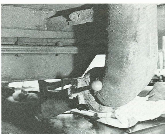
The tank's shut-off valve, located near an elbow, did not operate properly. When placed at a 90° angle to the pipe, it did not stop the flow of oil. The valve was later discovered to be defective.
