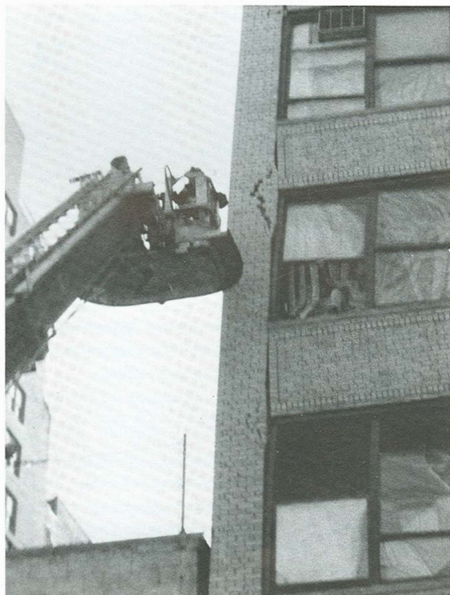
(Opposite page) From the exposure 4 side, floors could be seen hanging down inside the building. Photo by the New York Post (Right) Ladder companies quickly helped occupants leave via windows in the badly cracked front wall. Photo by Tim Brown
