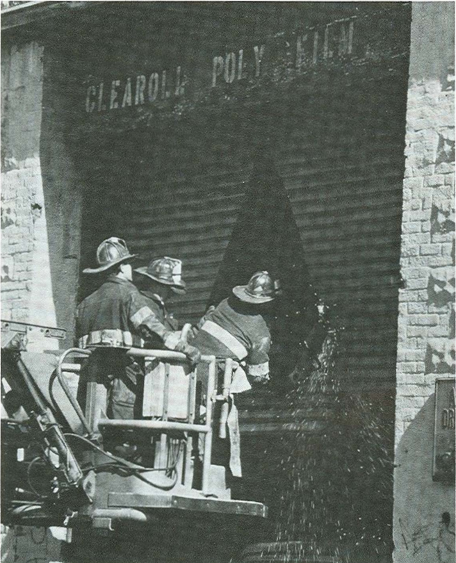
For one of the overhead, steel doors that faced onto the rear yard, only cutting would provide access. Photo by Jim Regan
