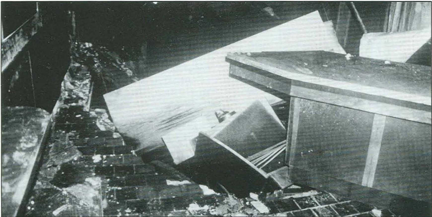
Moments after the last members left the store, the entire width of the store for the rear 40 feet fell into the cellar, with no prior warning--other than the presence of masonry!
