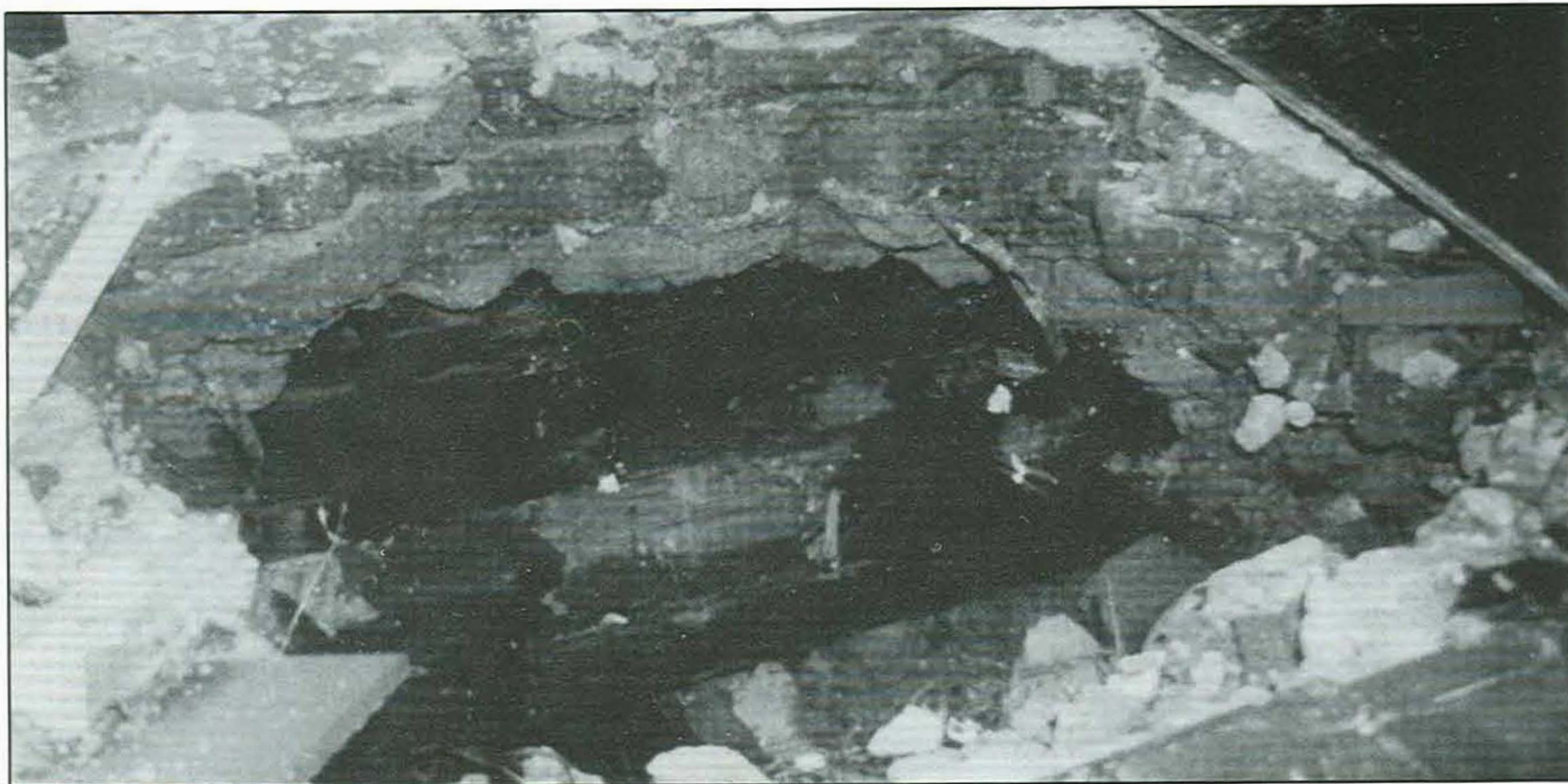
Firefighters breaching this 11 1/2 inch thick masonry floor (quarry tile, concrete, tile & terrazzo) found the floor supported by wood joists with heavy fire involvement. photo by Capt. John Norman
