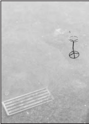
This knife-gate valve--which looks like a steering wheel--requires approximately 200 full turns to close.
