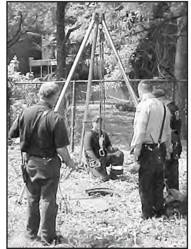
A tripod was raised over the manhole--as a high point anchor--in preparation for the rescuer's descent.
