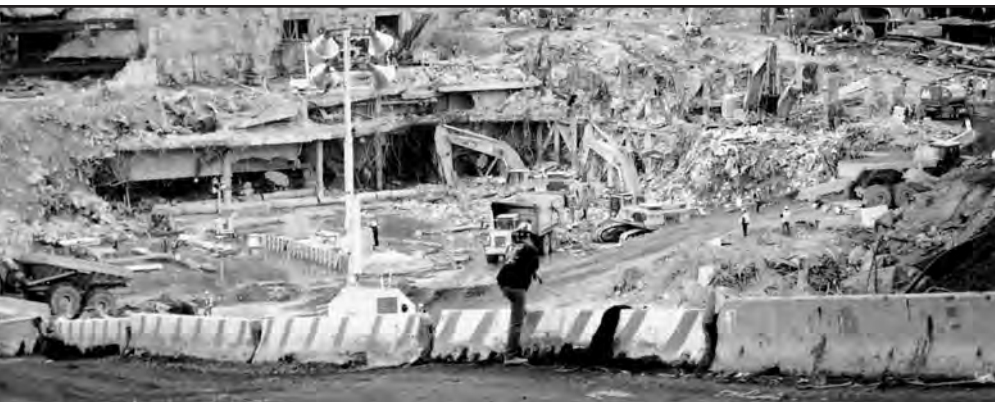
(Above) Fall protection--Jersey (cement) barricades along the Tully Roadway protected vehicle operators and recovery workers from fall injuries.
