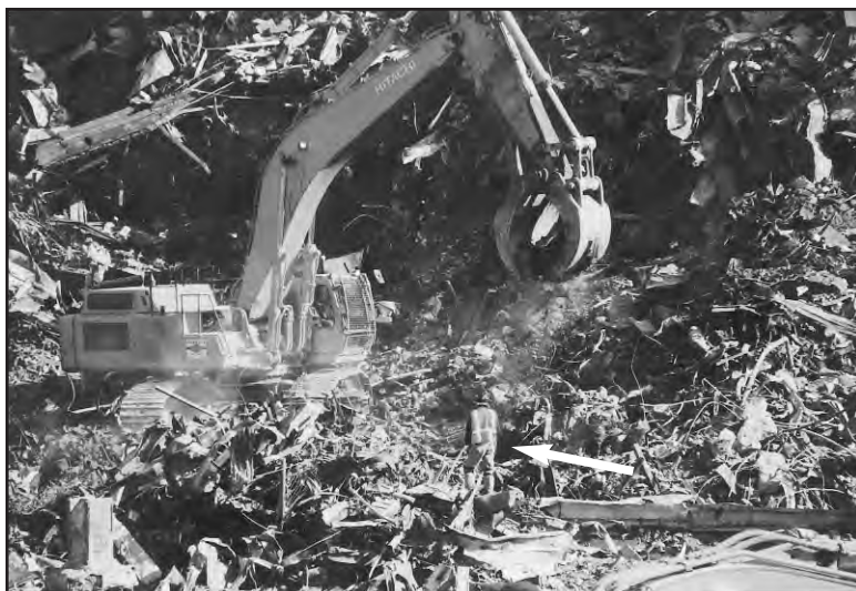
(Above) Lone spotter (debris removal observer) wore reflective vest (arrow) and stayed 50 feet from the operating radius of a demolition grapppler.
