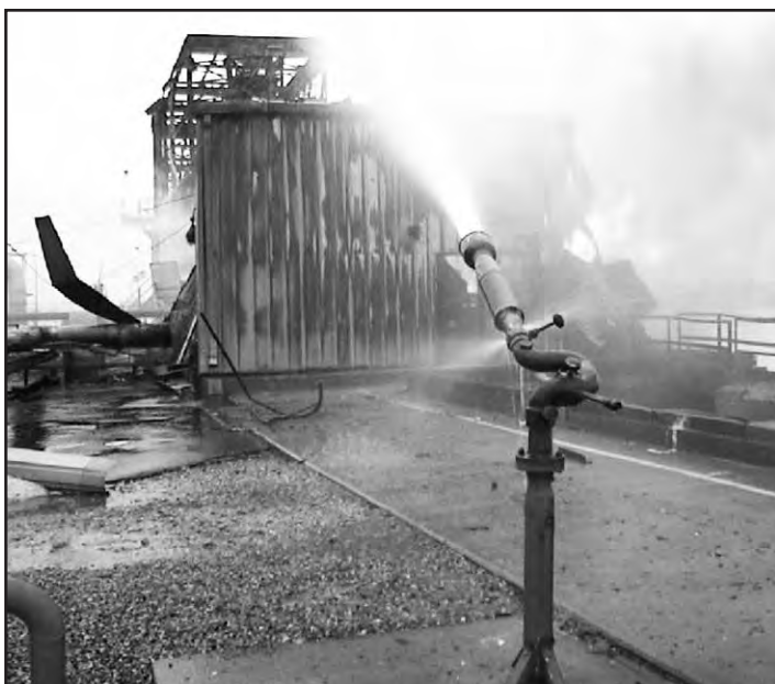
One of the fixed monitors provides a cooling stream on the remains of the destroyed pump house and piping.
