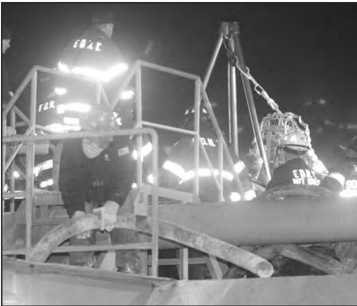
Con Ed employee breaks down 4½-inch flex hose as FDNY members remove victim via wire stokes and high-point anchor (tripod).
