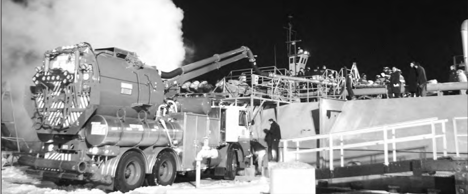
Con Ed vacuum truck in position on pier with suction boom, eight-inch aluminum extensions and 4 1/2-inch flex hose extending to the top of the barge.
