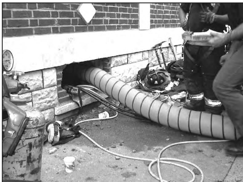
Units forced open a bricked-up cellar window to support the removal operation. Here, the ventilation duct and hydraulic hoses for the Stanley hydraulic blower, as well as electric lines and air monitor, are shown in the window opening.
