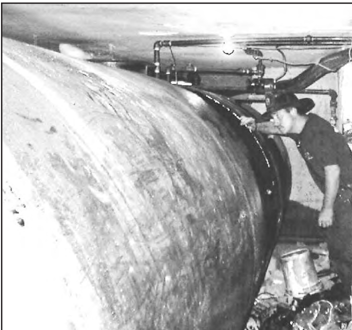
A view down the length of the 4000-gallon tank shows a rescuer surveying the scene. Note the minimal clearance (12 inches) between the concrete cellar ceiling and the lip of the manway the workers used to enter.
