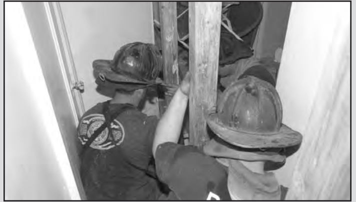
The shoring systems installed were a critical component to the overall success of this operation.
