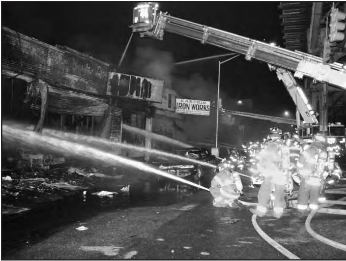
This photo reveals just how constricted FDNY operations were under the el. All members now are withdrawn from the collapse zone on the sidewalk and are operating from the safety of the street.
