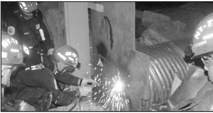
Team members had to cut through six inches of concrete. Here, they cut through an inch of steel in a large sewer pipe. It was a difficult operation because of the limited tools and equipment available to the members.
