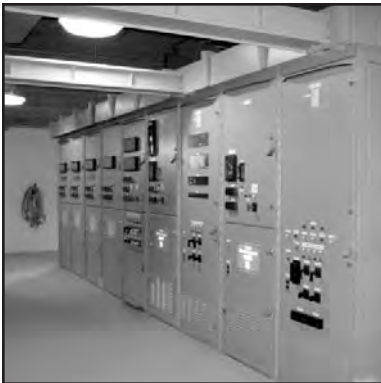
Photo #4--Circuit breakers are housed in locked cubicles to eliminate the chance of anyone casually entering these areas.
