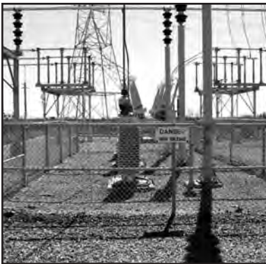
Photo #5--Lightning arrestors are found behind fences. Remaining outside of these fenced areas ensures your safety.
