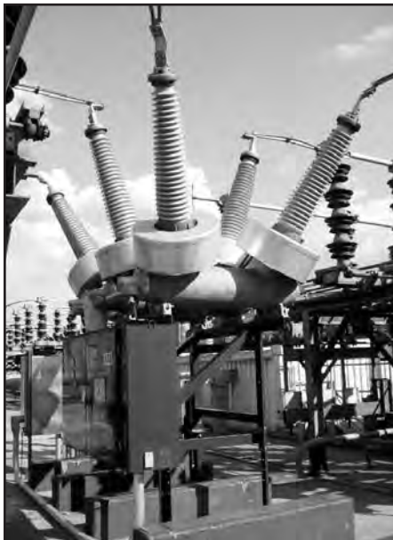
Photo #12--Sulfur hexafluoride gas is used to insulate and extinguish arcs in electrical components, such as circuit breakers.
