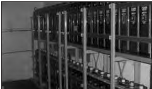
Photo #11--Each substation has two battery rooms, with each room holding 30 to 40 car-type batteries.
