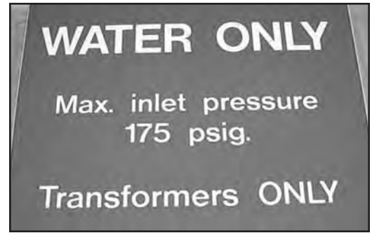
Photo #17--A sign at the siamese indicates the appropriate pressure.
