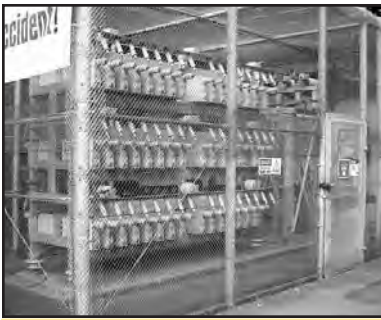
Photo #3--Capacitor banks reside in cages that provide a buffer zone between you and the exposed electrical conductors.
