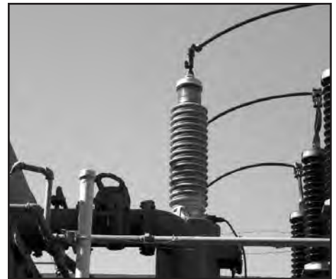
Photo #9--Oil-filled bushing.
