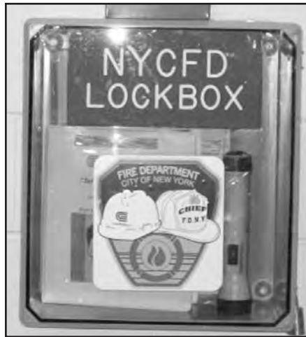
Photo #16--Con Edison maintains a lock box inside the substation gate for FDNY.
