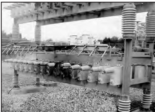
Photo #10--Edisol XT is a viscous-type of insulating oil used in capacitor banks.
