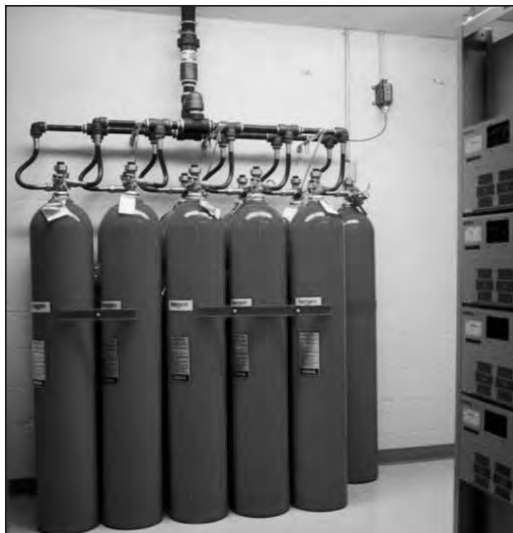
INERGEN (inside bank of cylinders shown) is a blend of inert atmospheric gases that boasts zero ozone depletion, zero global warming potential and zero atmospheric lifetime.
