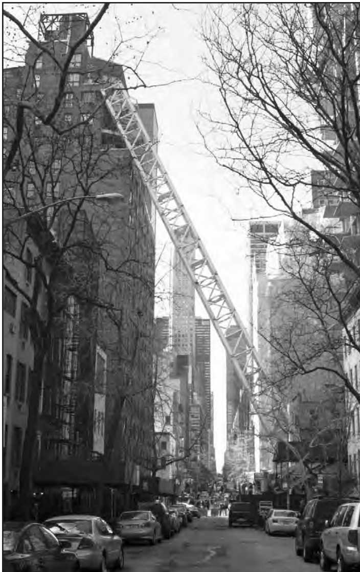
Photo #1--The 200-foot, 250-ton tower crane had broken away from a building under construction.
