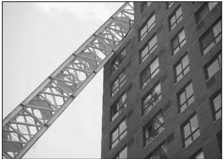
Photo #2--Tower crane leans on occupied, 23-story multiple dwelling at 300 East 51st Street.
