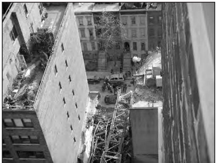
Photo #3--The crane cab and boom were severed from the tower and landed on the roof of a four-story brownstone.
