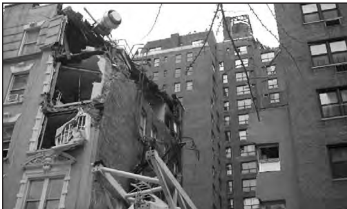
Photo #4--The rear wall of 944 2nd Avenue sustained heavy damage to the top floor.
