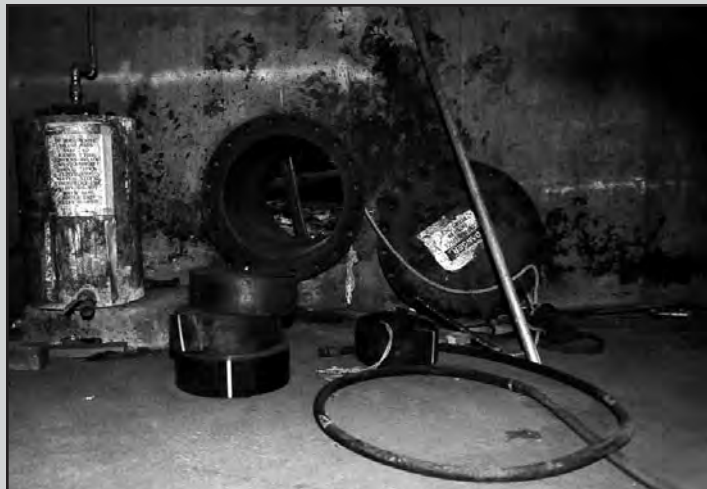
Base of the tank and the porthole within the building. The victim was partially within this porthole and exited here. Exterior tank operations took place at this location.
