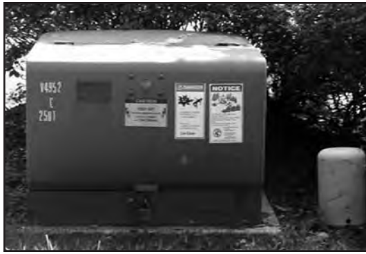
Photo #4--Pad transformer.
