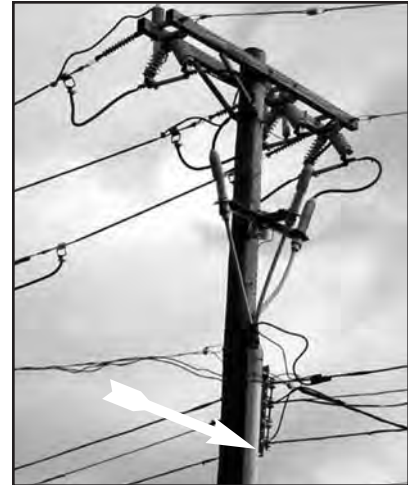
Photo #1--Riser pole is supplying high-voltage lines (arrow).
