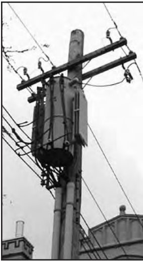
Photo #3--4kV transformer supplying secondary risers.
