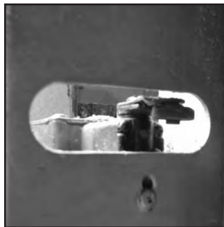
Photo #19--Gate switch.
