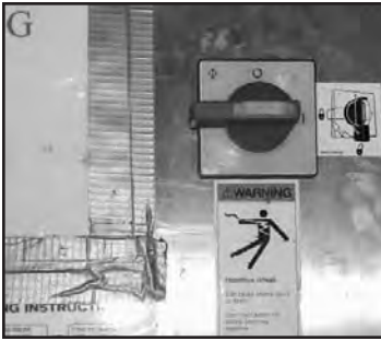
Photo #13--Alimak power switch car.
