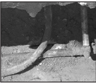
The electrical conduit and gas line that caused the explosion.
