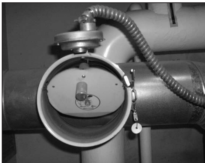
The draft inducer pictured is a device to assist with the drafting of flue gases up the chimney. The counterbalance weight pictured on the right side opens the flap to create a draft. The electrical component above is a roll-out switch. The switch will shut down the boiler if it becomes overheated, indicating that hot flue gases are escaping through the inducer.
