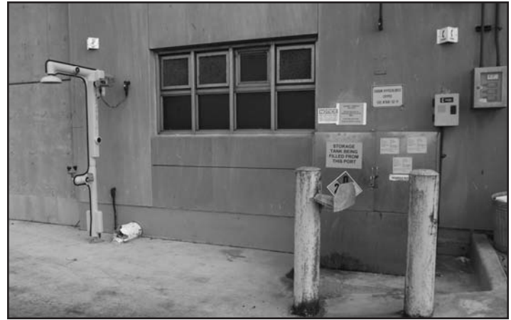
Sodium hypochlorite solution delivery area.
