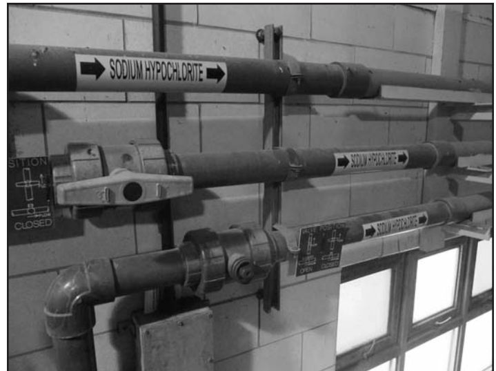
Labeling and signs denoting product identification, flow direction and valve positioning information.
