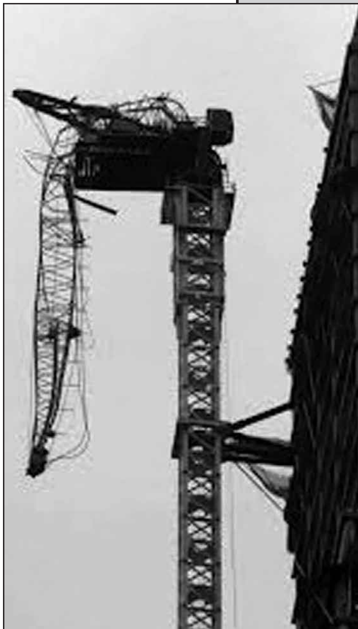
Crippled crane at West 57th Street, Manhattan (Box 916), dictated a four-alarm response by FDNY units during the storm.
