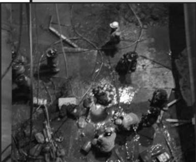
Plywood was used to provide a work and walking platform atop the Bull's liver.
