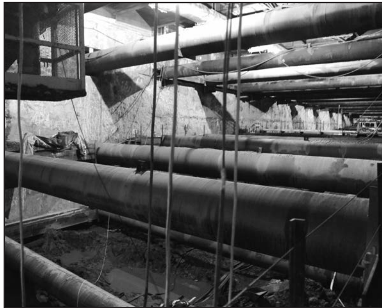
Large-diameter steel pipes, acting as lateral shoring struts for the excavation walls, were used as high points.
