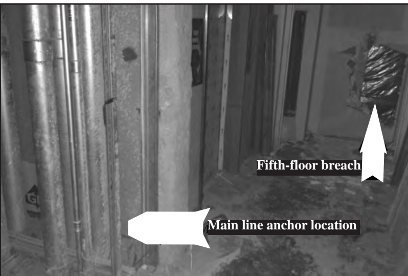
Photo #5--The main line was anchored to six-inch-diameter steel conduit on the fifth floor. This was eight feet back from the breached wall. This breach is where FF Baron entered the shaft. The main line and safety line were operated on this floor.
