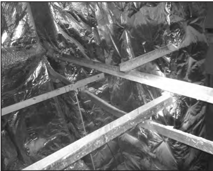
Photo #3--Grids of two- by two-inch, steel angle-iron are affixed throughout the mechanical shaft. They support the air ducts on which the worker landed.
