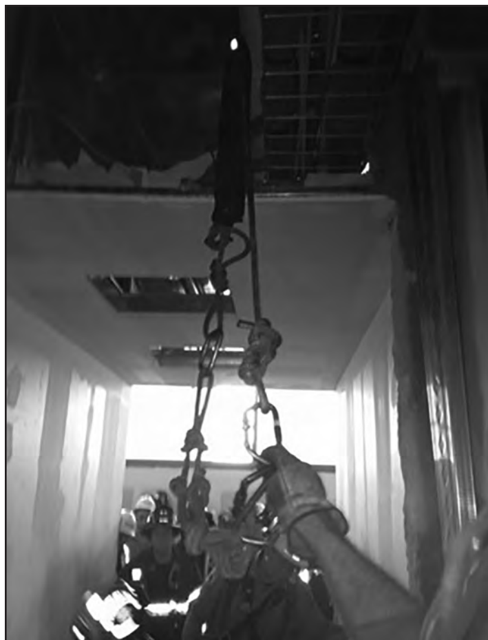
Photo #6--This photo was taken after the patient was removed to the ambulance. The service panel opening where Ladder 78 first made contact with the injured worker is visible in the background. The main line is on the left in the photo. Note that the main line was attached to a two-legged bridle. The bridle was attached to the LSP (Life Support Products) Half Back Extrication Device at two points. This practice of using a bridle spreads the patient's weight out and can make a device less constricting. Also on the main line is an anti-chafing sleeve that slides down when the rope no longer is under tension. The safety was connected to the LSP at another attachment point. The LSP Half Back Extrication Device is a tool that can be applied to a patient to provide rapid immobilization and vertical lift/lower extrication. It is a padded, full-body harness that uses clips to attach it to the patient. These clips allow the rescuer to apply the device with minimal patient movement. The Half Back also has a rigid insert with a head immobilizer for use when trauma is suspected.
