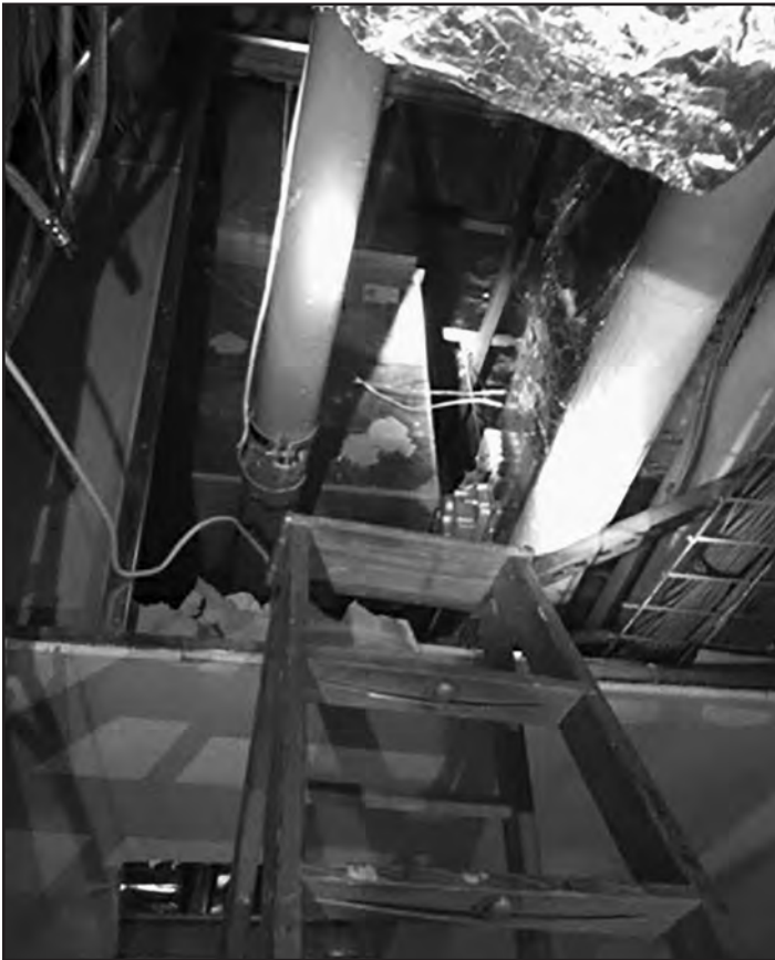
Photo #8--The route through which the worker was lowered left little room to spare. A stokes basket would not fit past the obstructions. The man was guided physically during the entire lowering operation.
