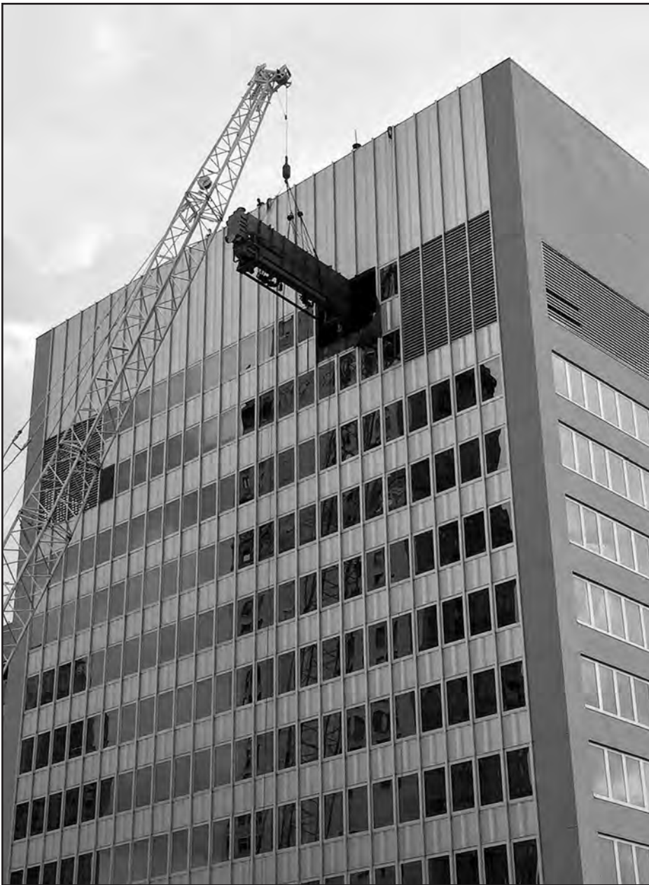
Crane control of the chiller is lost. The result is damage to the building--bouncing off several floors, breaking window glass--before the chiller fell to the ground on Madison Avenue, causing yet more damage.
