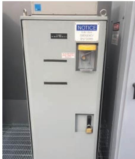
Emergency Power Off (EPO) button shuts off electrical power, as well as gas flow within a fuel cell system. Photo by author
