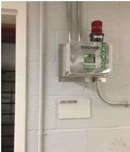
Fixed gas monitor with red warning light outside enclosure, harboring natural gas distribution piping for fuel cell installation. Photo by author
