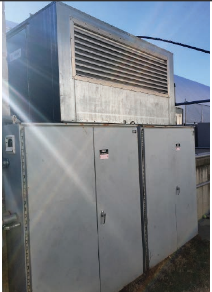
Photo #4—Natural gas-powered generator. This is the primary fan unit of North Shore Indoor Sports, Bayside, Queens. There will be a knife switch located on the unit.
