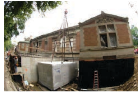
Fuel cell system being installed in the basement of the Madagascar building at the Bronx Zoo. New York Power Authority, Energy Technologies https://www.nypa.gov/services/profiles/Bronxzoofuelcell.htm
