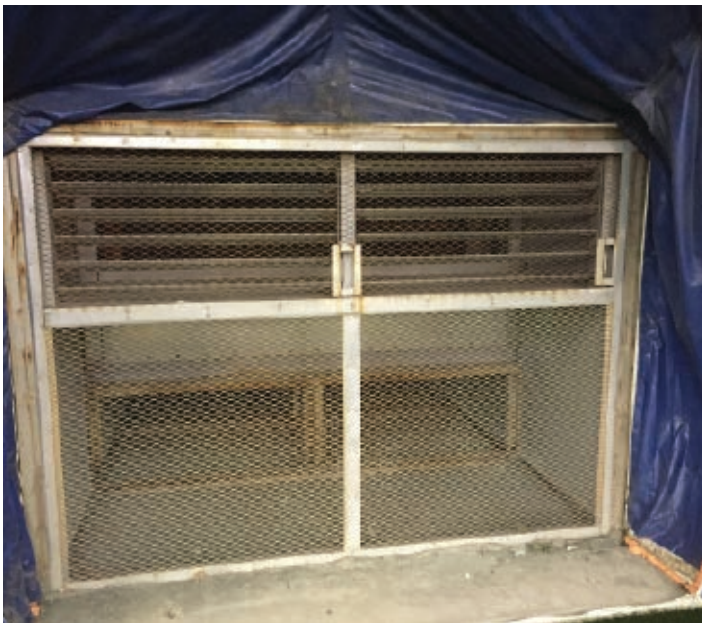
Photo #3—An exhaust fan in an air-supported structure. This permanent fan exhaust system is located at North Shore Indoor Sports, Bayside, Queens.
