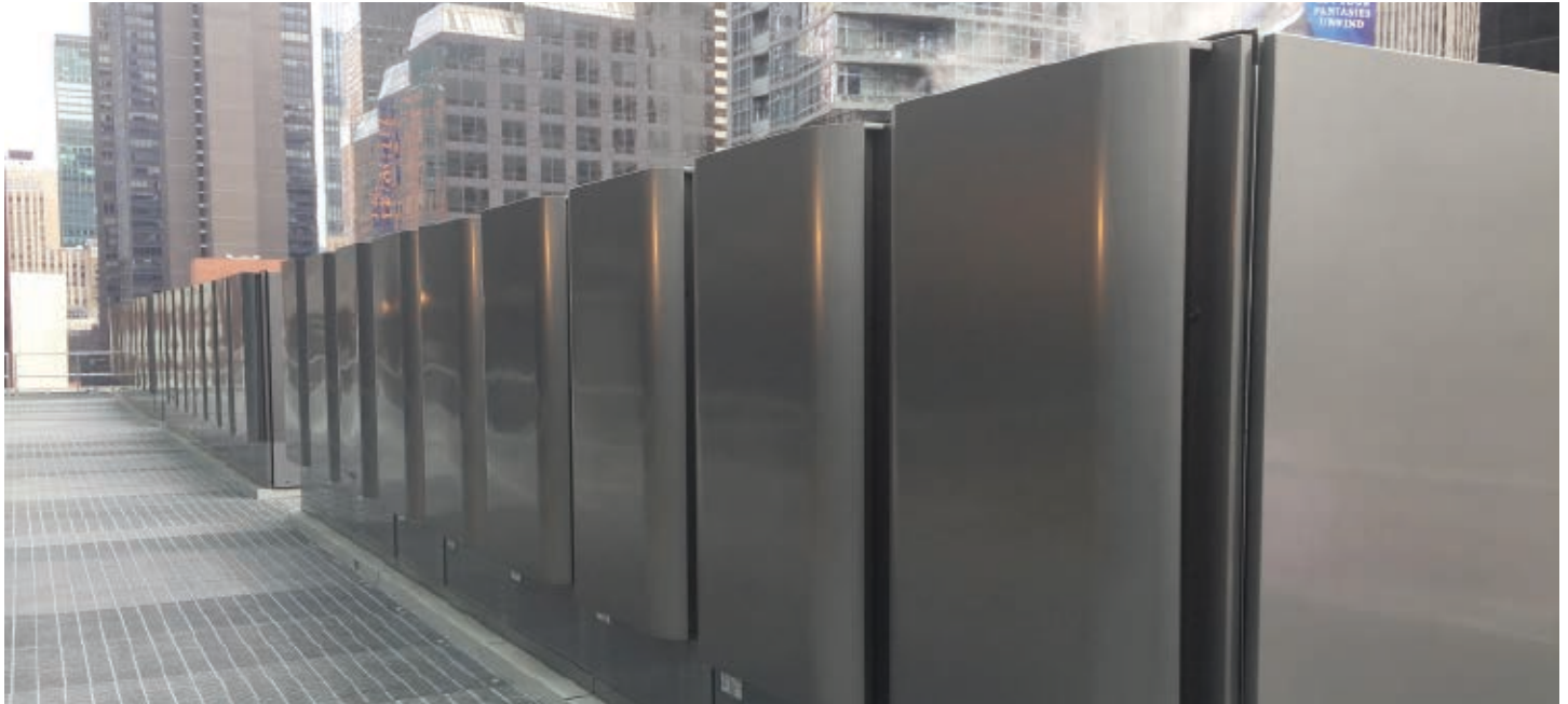
Fuel cell installation using natural gas, located on setback roof at Morgan Stanley building in midtown Manhattan. Photo by author
