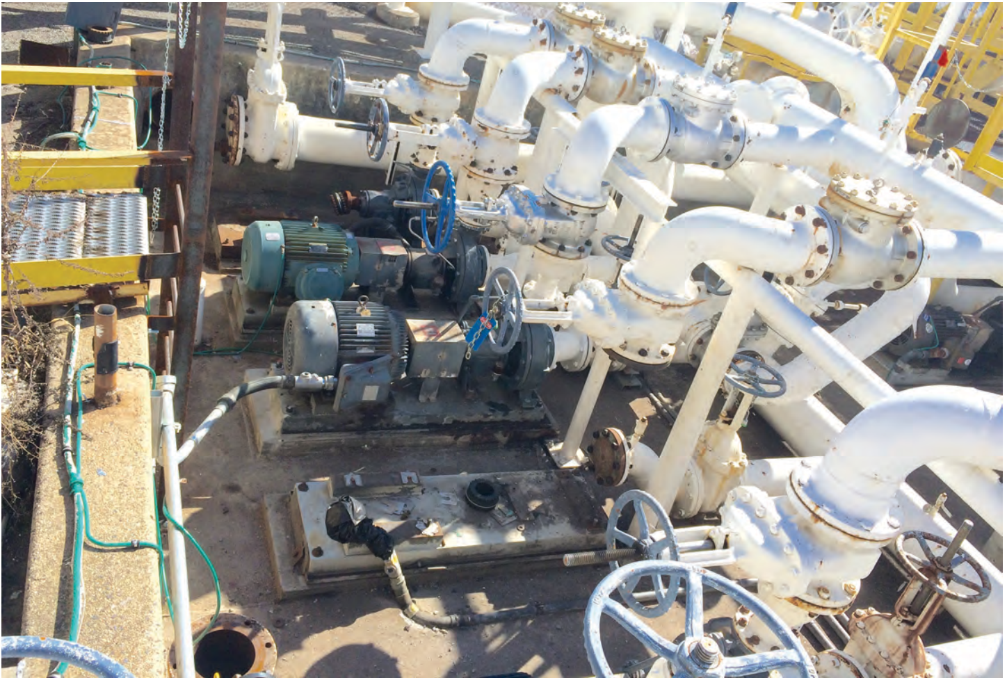
Pump B now is removed and out for repair. The fixed vertical ladder at left is how FDNY members gained entry. The two OS&Y valves closed to stop the leak are above and behind the missing pump.
