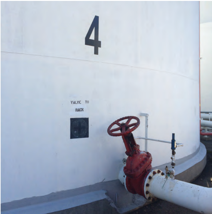
The OS&Y valve used to control tank 4. It had been closed by the plant operator before FDNY's arrival, but there was an estimated 1,600 gallons of product still in the piping.
