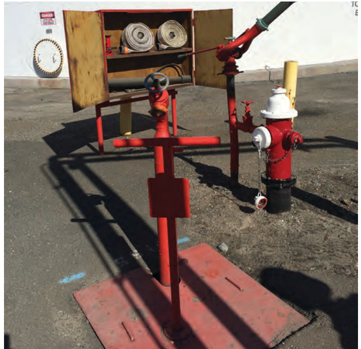
Plant firefighting stations are found throughout the area. The fixed monitor with the hydrant is used for water streams. The outlet in the foreground has an orange cap, denoting it as supplying foam solution to be used with the hose and foam nozzle in the background.
