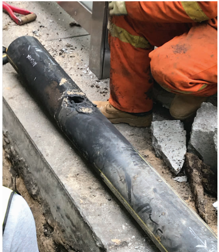
Damaged plastic gas supply line. Photo by Lieutenant Clifford Freer, Haz-Mat Training, FDNY.
