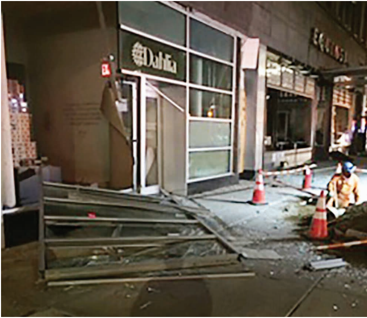
Explosion damage to the building.
