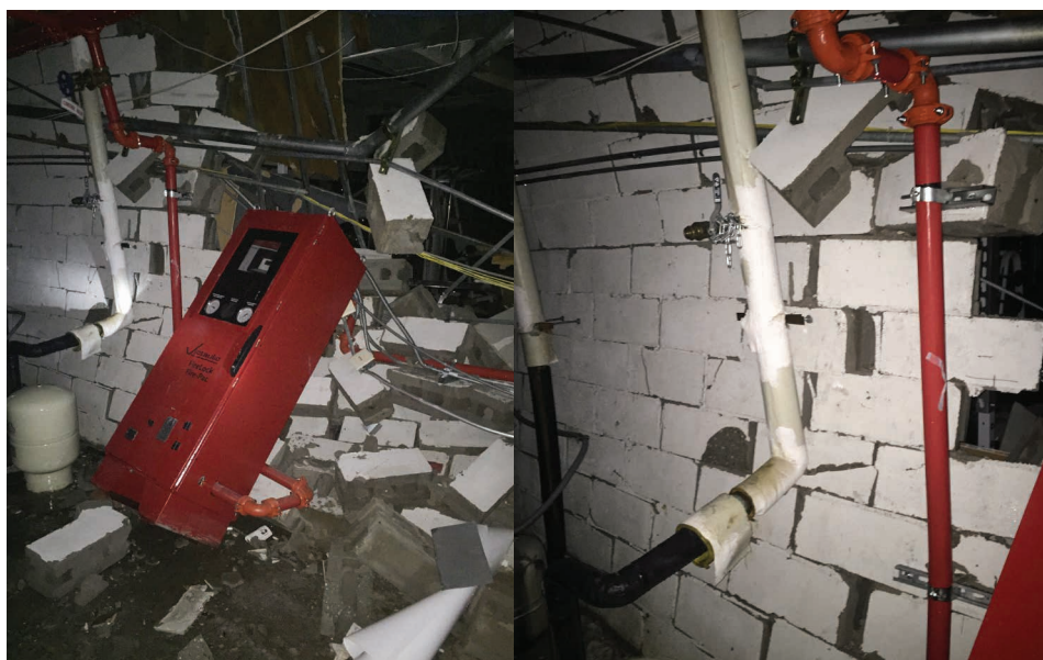
Wall and ceiling damage in basement.
