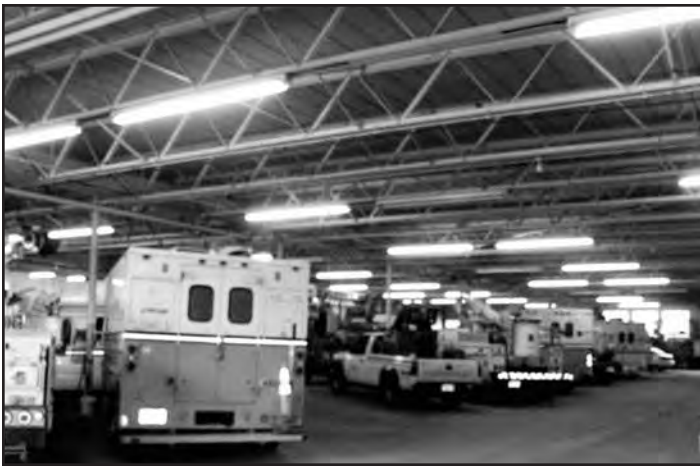
Photo #6--Trusses may be unprotected over areas housing significant fire loads.
