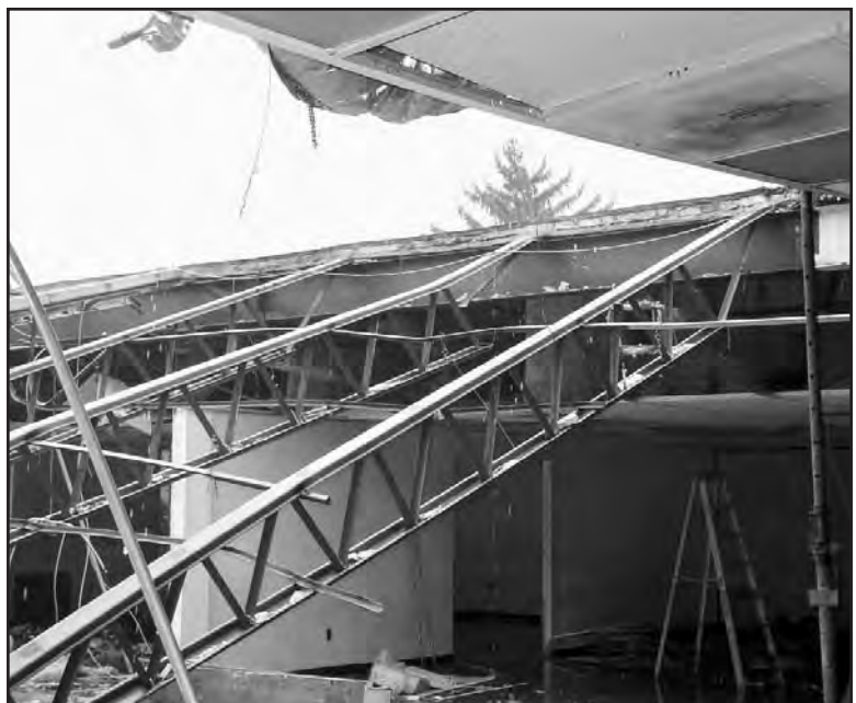
Photo #5--Trusses often collapse under normal loading conditions in the absence of fire. Here, snow was the culprit.
