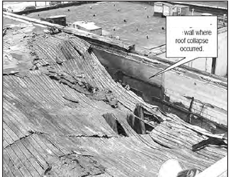
Photo #4--This truss-supported roof collapsed due to fire.
