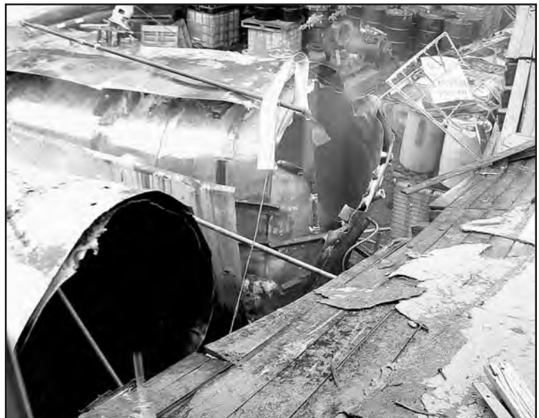
The storage tanks were made of double-walled steel, with insulation between the inner and outer walls. When the tanks exploded, they failed at their ends. The insulation continued to burn. Note how the tongue and groove roof flexed and bent, but did not fail.
