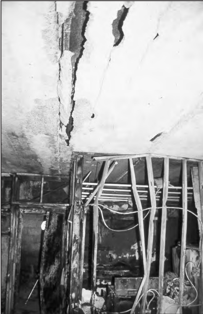
Temperatures had to have reached 3000 degrees to cause this damage to the pre-cast concrete ceiling at the Vandalia Avenue fire apartment. This occurred within the 25 minutes it took a hand-line to be advanced the 45 feet to the door of the apartment.
