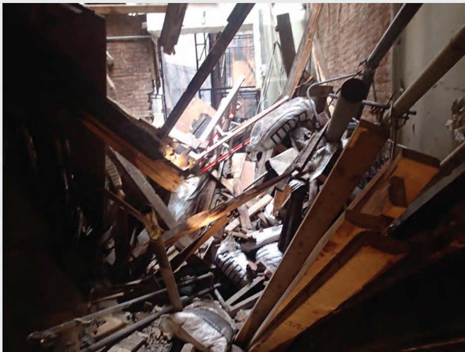
View from Above. FDNY members are positioned on the second floor, above the debris pile, monitoring the movement of the collapse.
