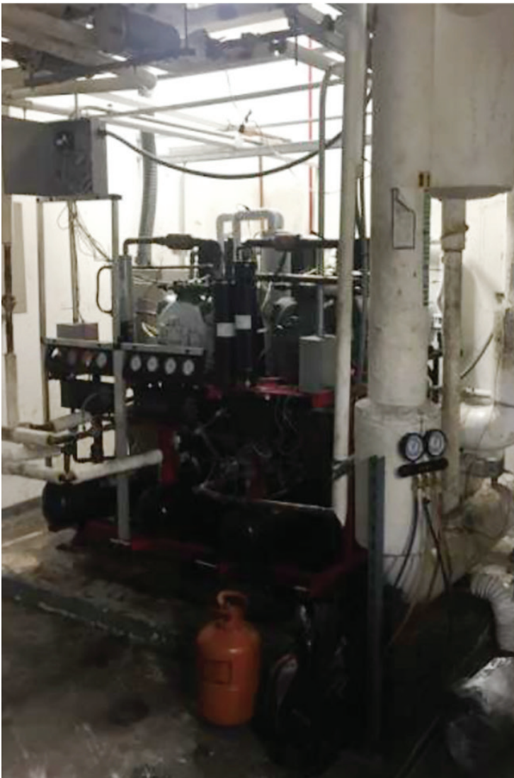
Photo 2—Large air-conditioning system located in the basement of the library.
