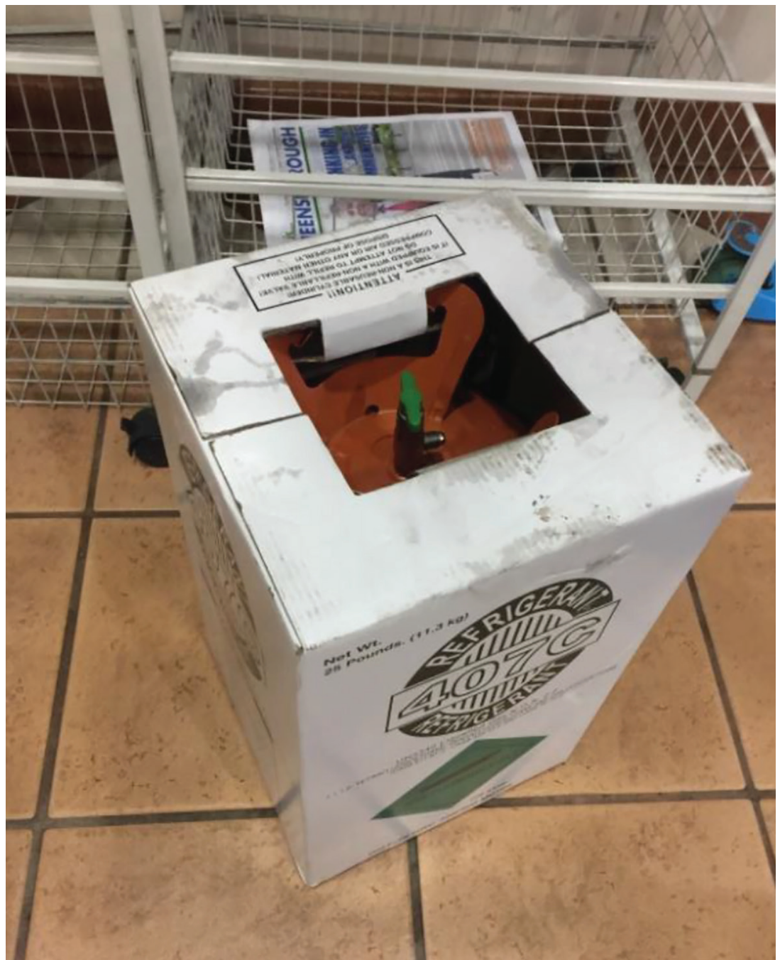
Photo 1—Container taken from basement to confirm refrigerant.
