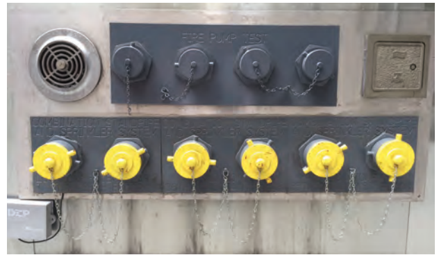
Photo 2—A tiered standpipe system requires engine company chauffeurs (ECCs) to connect to the proper siamese.
