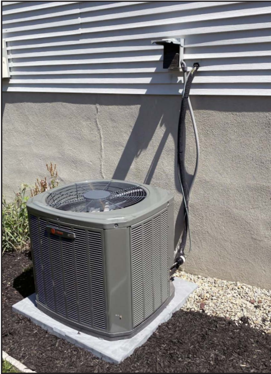
This is a condenser where the heat is discharged from the refrigerant. The electrical disconnect switch (located on the exterior siding) can be pulled to kill power to the system.
