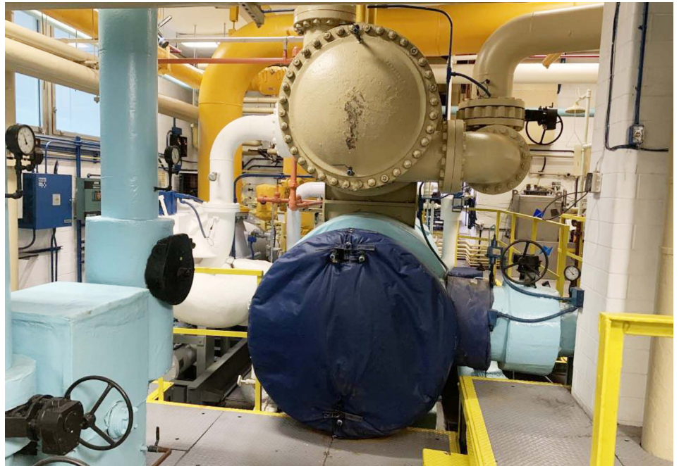
Commercial chiller plant
