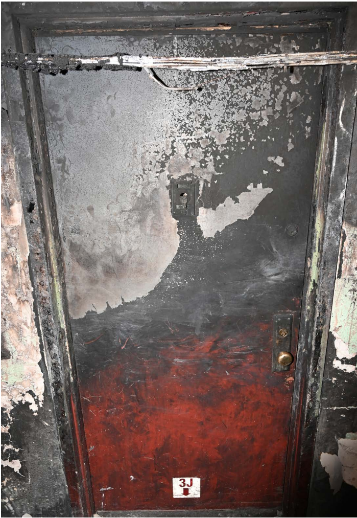
The door to Apt. 3J, which is across the hall from Apt. 3N (fire apartment) and several feet closer to the attack stairway. Six 10-45s, including two children who perished, were located in Apt. 3J. (Photo credit: Bureau of Fire Investigation)
