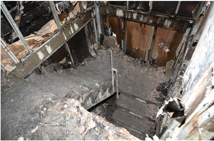
The “duplex-down” staircase in Apt. 3N, the fire apartment. (Photo credit: Bureau of Fire Investigation)
