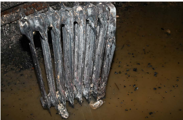
The FDNY Bureau of Fire Investigation officially determined that a space heater in a lower-level bedroom (exposure 3 side) of Apt. 3N caused the fire. (Photo credit: Bureau of Fire Investigation)
