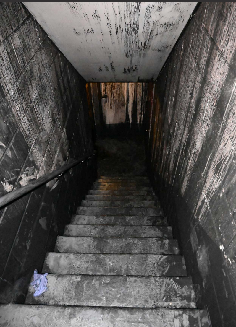
Stairwell B (attack stairs) looking down from the eighth floor to the seventh floor. (Photo credit: Bureau of Fire Investigation)
