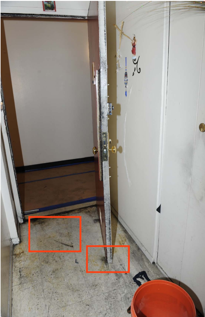
An exemplar photo of an apartment door at Twin Parks that was stuck open in an unburned apartment. The black scuff marks on the floor indicate that the door was contacting the floor. This can occur if additional floor tiles are installed over the original flooring. (Photo credit: Bureau of Fire Investigation)
