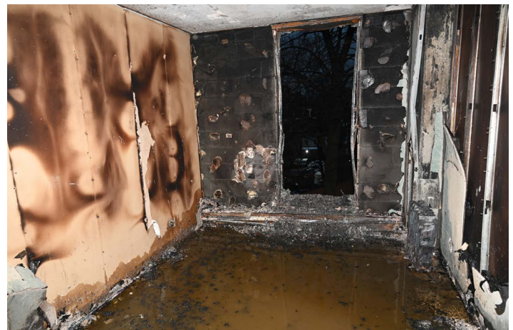
The lower-level bedroom where the fire originated in Apt. 3N. This room is on the second floor. (Photo credit: Bureau of Fire Investigation)
