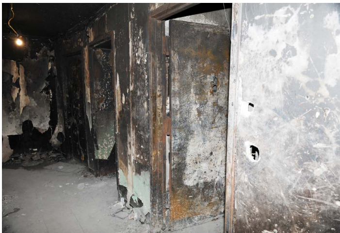
The door to Apt. 3N, the fire apartment, from the third-floor public hallway. (Photo credit: Bureau of Fire Investigation)
