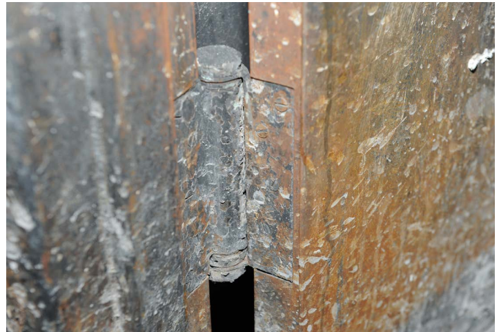
A spring-loaded hinge on the self-closing door to Apt. 3N. This door failed to close as occupants fled the fire apartment. (Photo credit: Bureau of Fire Investigation)
