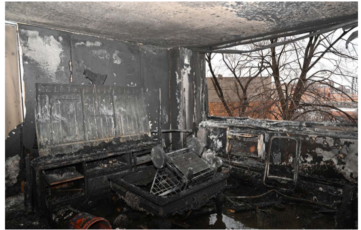
The living room on the upper level of Apt 3N, facing the exposure 3 windows. This room is on the third floor. (Photo credit: Bureau of Fire Investigation)
